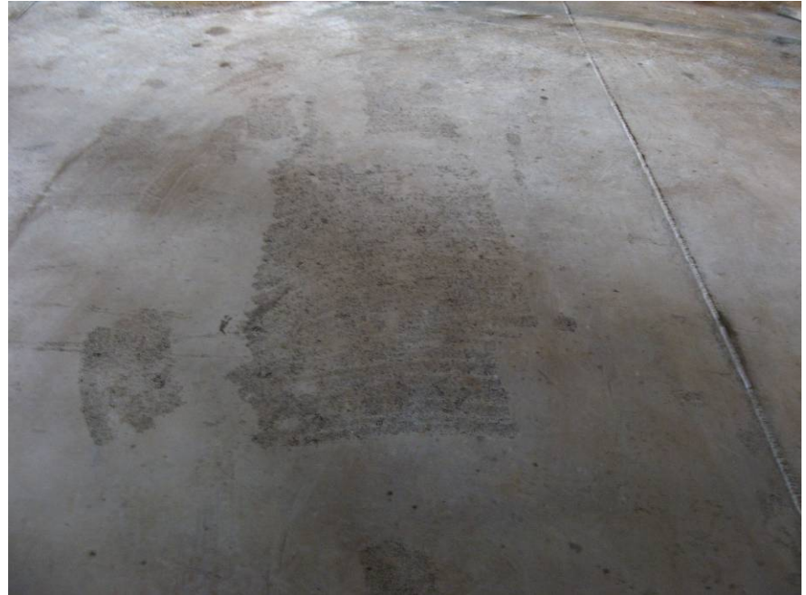
Corrosion pattern following grinding marks on floor
