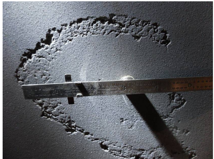
Indirect lighting with LED flashlight reveals corrosion
